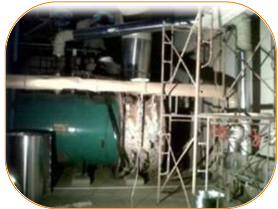
Steam Tank Installed at Gatron Industries Ltd
