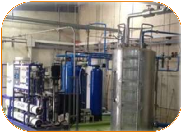
Machinery Installed in YAMAHA Motor Company
